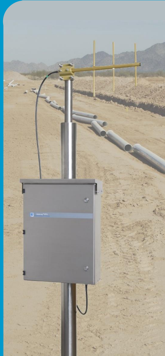
AutoLog® Cathodic Protection WRMU
